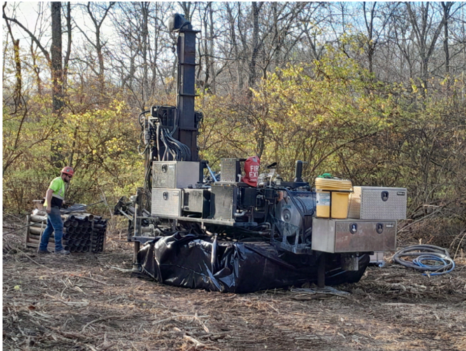
Figure 2. The sonic drill rig used to drill the soil borings TRN-1 to TRN-7 from November 7-14, 2022.
